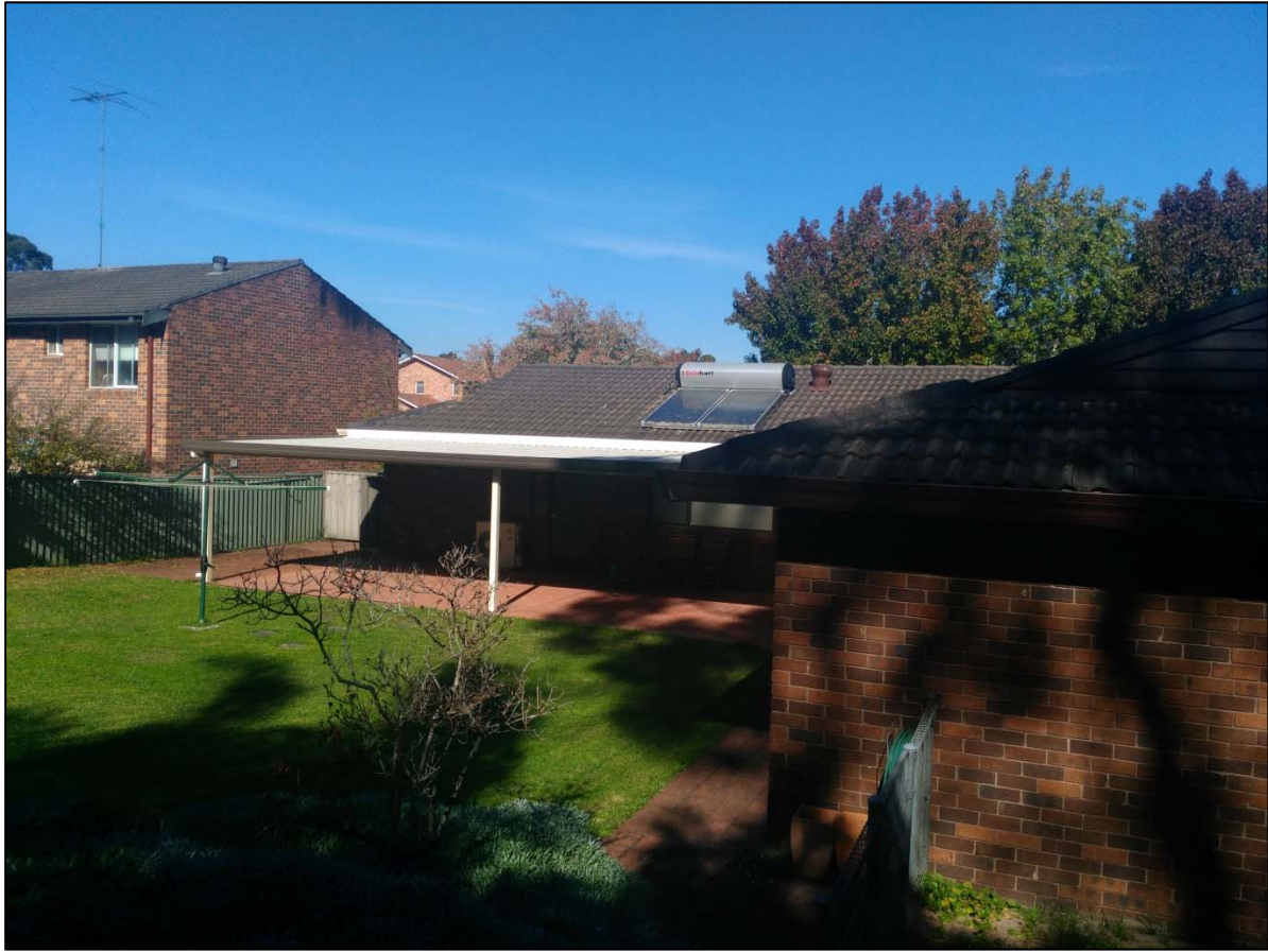
Photograph 1: View from the back of 27 Dawes Avenue – Building in relatively good condition. Roof tiles showed signs of minimal weathering, however corner of eave (pictured to the right) showed some signs of degradation (i.e. flaking paint and guttering had some rust build up).
