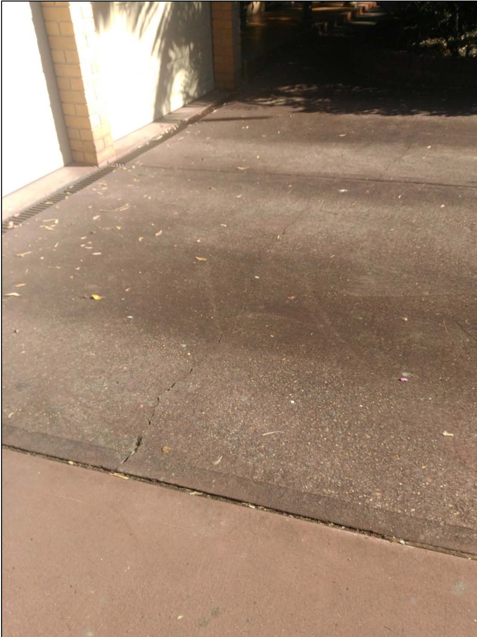
Photograph 5: Minor cracks observed in concrete hardstand.
