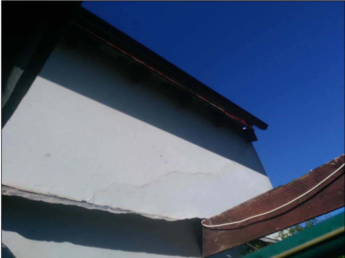
Photograph 2: Signs of weathering shown on a site building; exposed metal capping (in moderate to poor condition), external cracks in brickwork, overhead wooden beams show some signs of weathering and rust build-up was observed on guttering.
